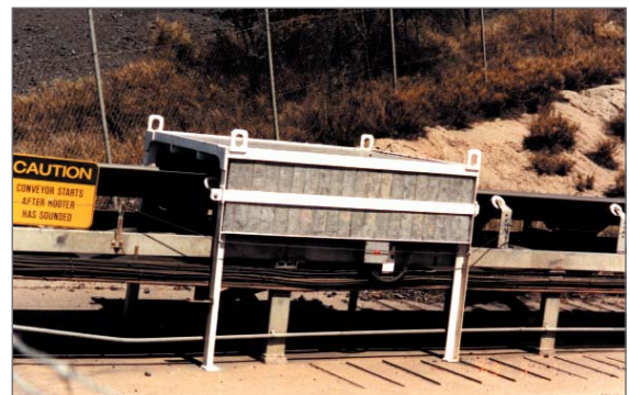
COALSCAN 1500: an analyser is installed under the belt. Above the belt is lead shielding.
